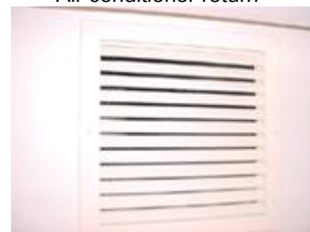
Air conditioner return
