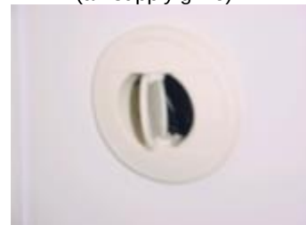
Air conditioning vent (air supply grille)
