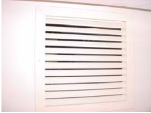
Air Conditioner Return on the face of the V Berth storage area
