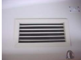
Air Conditioner Vent in the Main Salon
